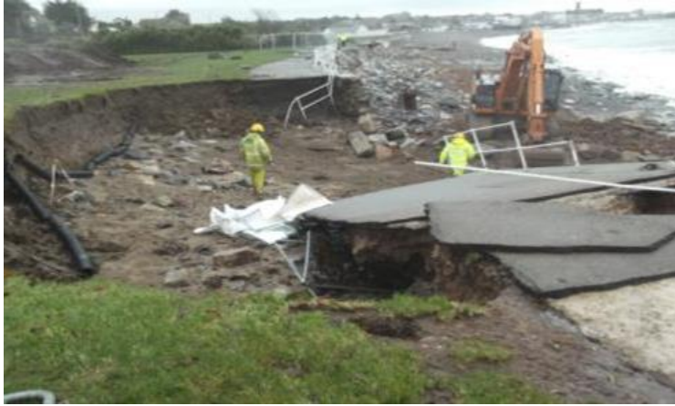
Figure 5: Erosion storm impact at Newlyn Green
