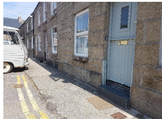
Figure 6: Property Flood Resilience at Tolcarne
